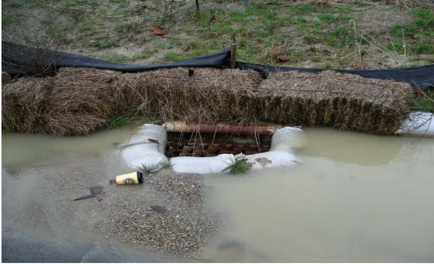
Sandbags around a storm drain helps keep sediment from entering the drain.
